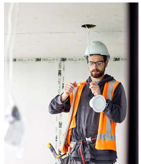
Making sure learners uphold quality workmanship and are working to industry standards.
